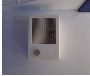
Service Area Heater
