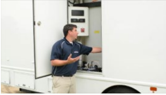
Water Filter in Unit.
