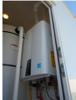
Plug in Back Water Heater
