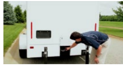
Accessible 4" Clean Out Port.
