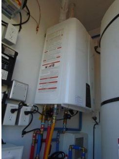
Front Water Heater
