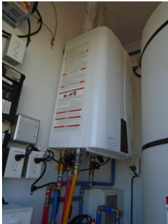
Plug in Front Water Heater
