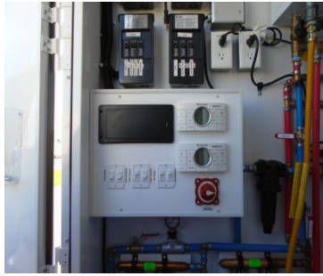
Battery Disconnect in unit
