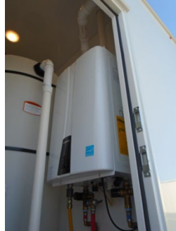
Back Water Heater
