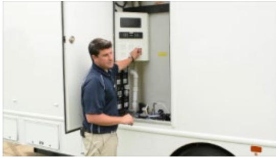
Battery Disconnect in unit
