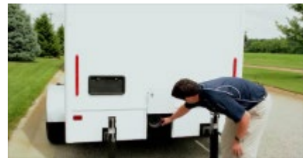
Accessible 4" Clean Out Port.
