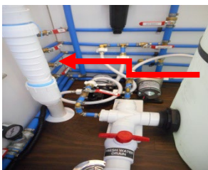
Location of Urinal Shut Off Valve in Service Area.
