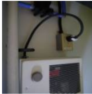
Service Area Heater
