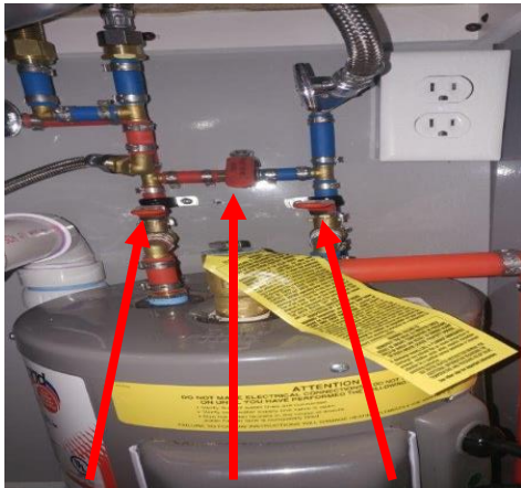
Inlet Bypass Outlet
