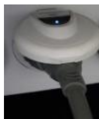
Check Blue Light on Trailer
