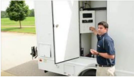
Battery Disconnect in unit
