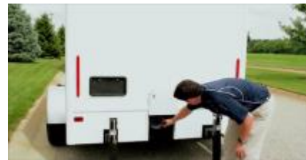
Accessible 4" Clean Out Port.
