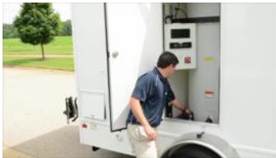
Pressure Gauge in Unit.
