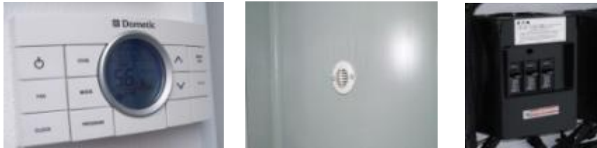
1. AC/Heat Control Panel 2. Thermostat Sensor 3. AC Breaker
