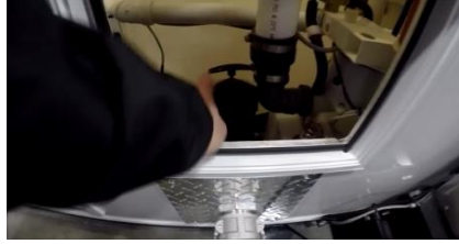
Accessible 4" Clean Out Port.
