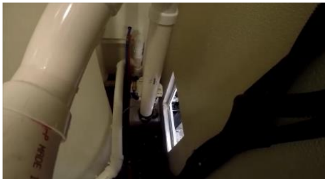
Black Water Tank
