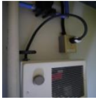
Service Area Heater
