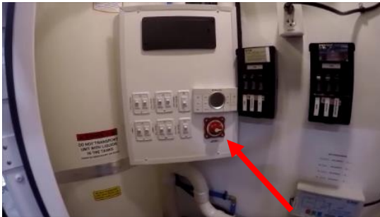
Battery Disconnect in unit
